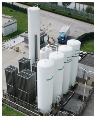
On-site gas generation
