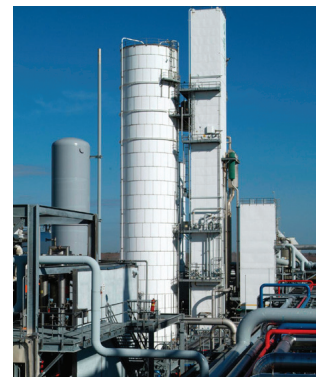
Large air separation unit and pipeline system
