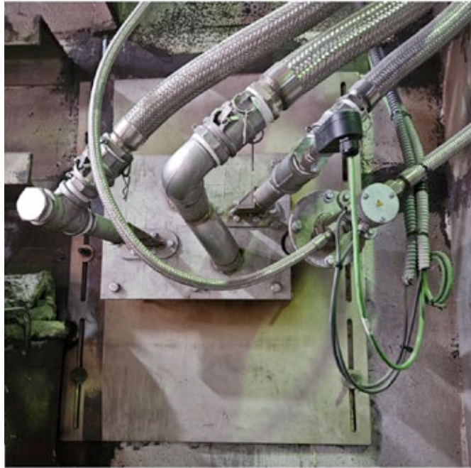
Figure 4: HTHB mounted on a reverb furnace wall.
